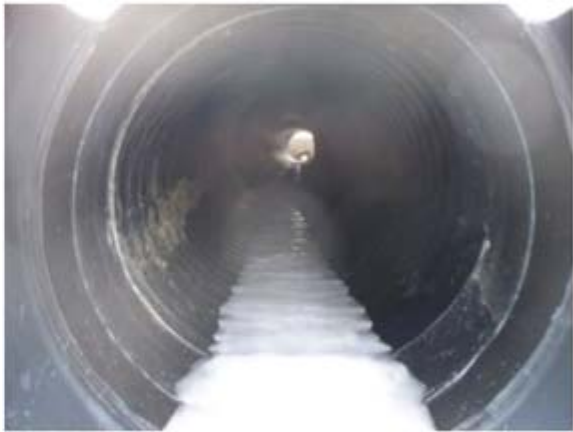
Contractor poured a concrete cradle Around the bottom and sides of pipe For rigidity.
