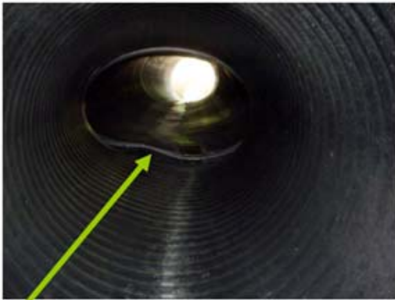
This pipe squashed and pushed Up from the bottom
